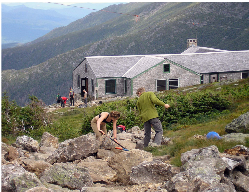
The RMC trail crew at work reconstructing the Crawford Path; AMC's Lakes of the Clouds hut in the background. Bob Drescher photo.
