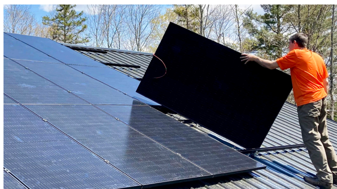
Top, the south-facing slope of Stearns Lodge's new metal roof; above, Mike Flanagan of DTL Electric, tilting a solar panel into place. Photos by J. Maddock, Sally Micucci.
